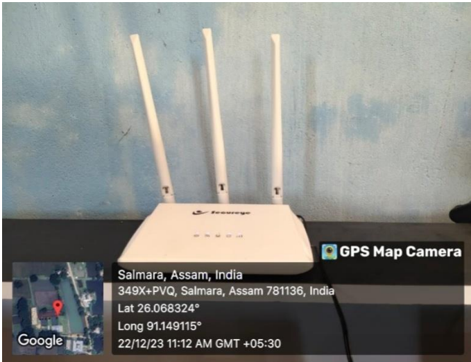
Photo 7: Router for internet connection
